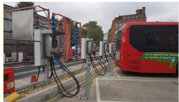
▶ Plug-based charging at Waterloo Garage. Source: Go-Ahead London
