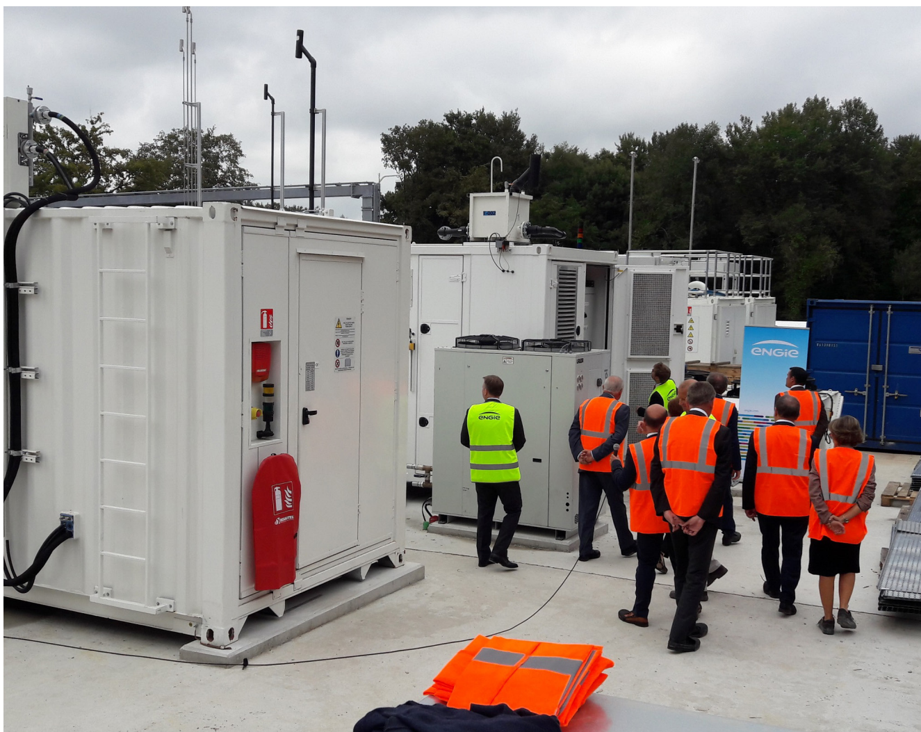
► Hydrogen refuelling structure facility in Pau, France
